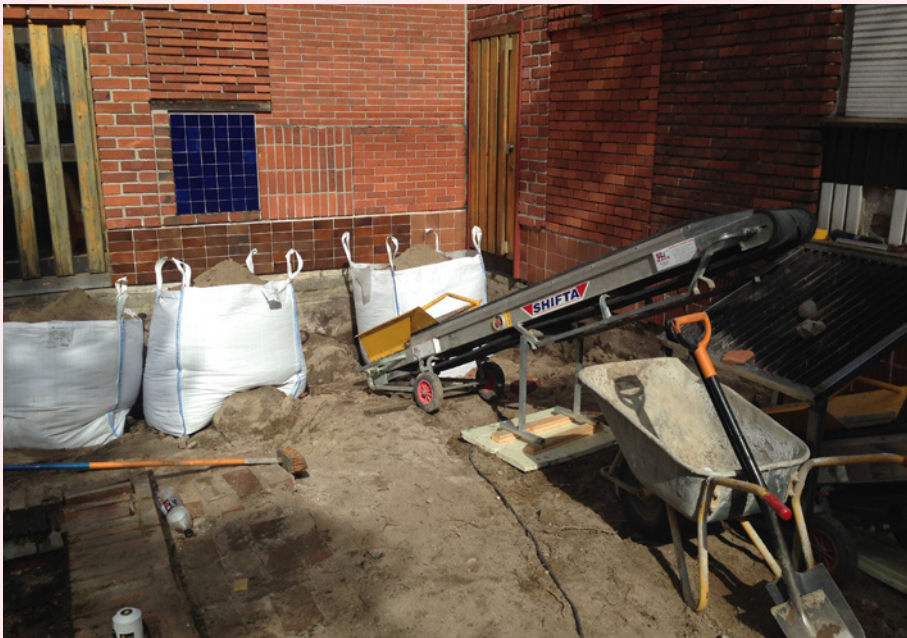
The Muuratsalo Experimental House 2015. During the restoration of the patio. All the bricks on the patio floor were numbered and stored. The ground substance was changed from fine sand into gravel. Photo: Tommi Lindh.
