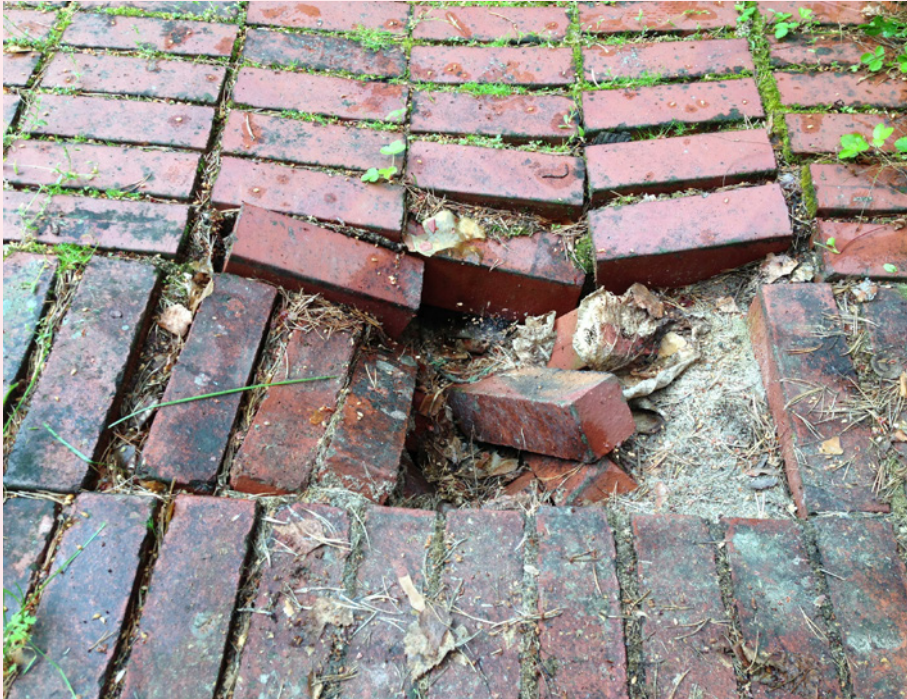
The Muuratsalo Experimental House 2013. Before the restoration of the patio. As seen in this picture areas of the courtyard had collapsed due to the soil underground having moved elsewhere with rainwater. Photo: Tommi Lindh.
