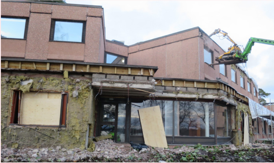
Hanasaari Swedish-Finnish Cultural Centre 2015. During the removal of the outer concrete panels. Photo: Architects Kirsi Korhonen and Mika Penttinen.
